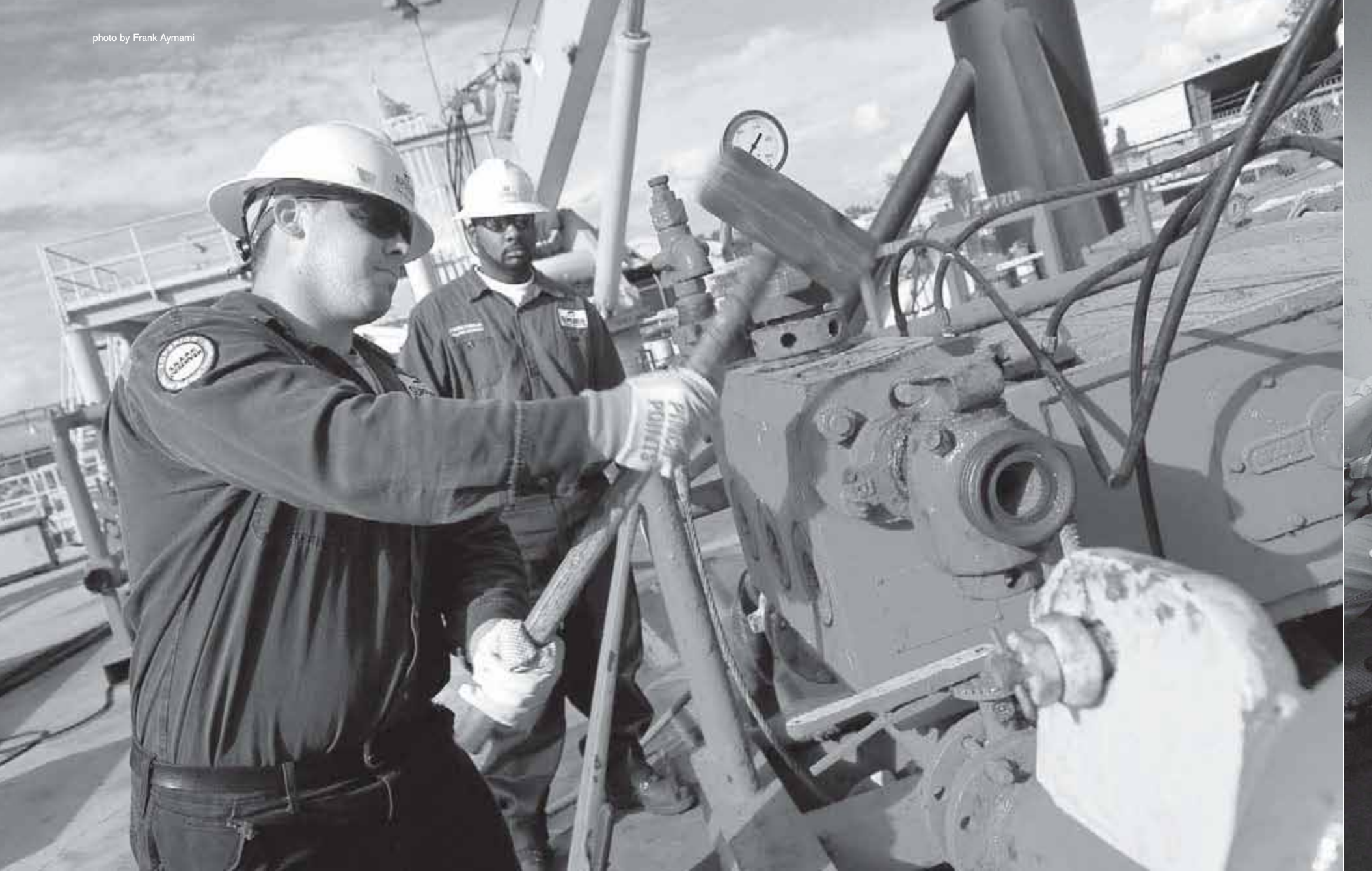
Pump operator Tim Miller, left, and crane operator Jerome Fobb Jr. prepare a pump at Superior Energy Services' Harvey facility.
