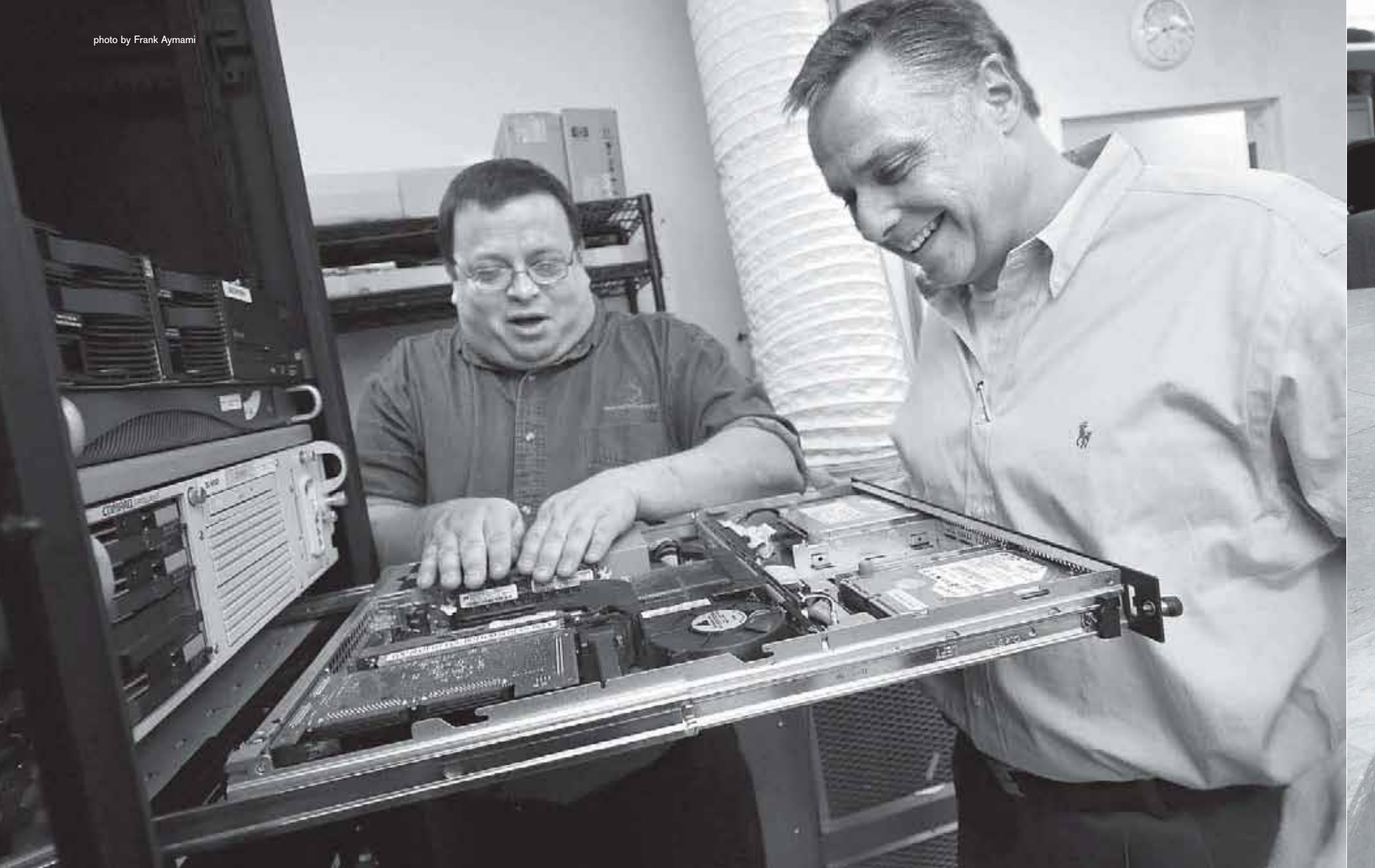
Network engineer Robert Breland, left, and CEO Joey Auer work in Diamond Data Systems' server room.
