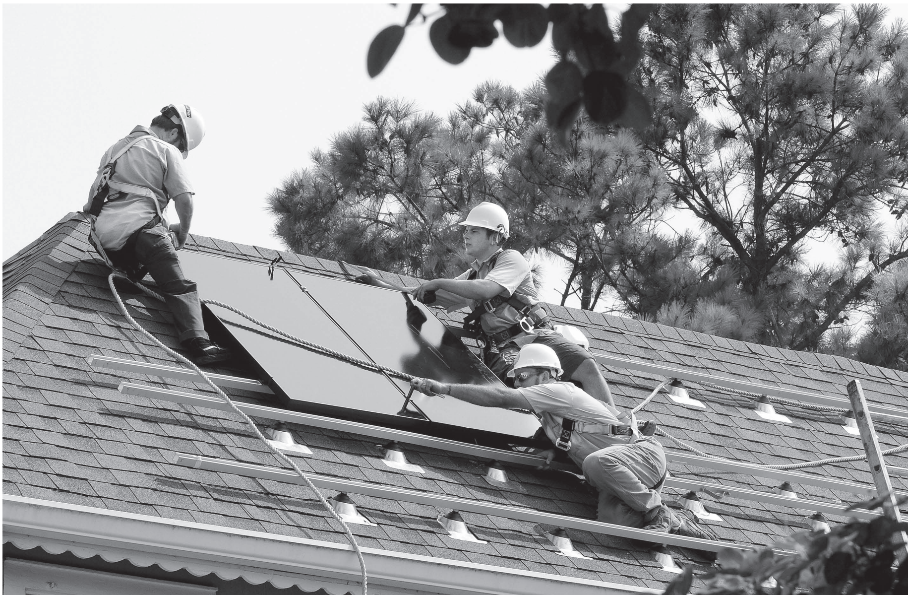
SouthCoast Solar employees, from left, Tim Coats, Micah Galy and Issac Wright, install a solar panel on a customer's roof.
