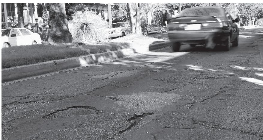
The Federal Highway Administration's South Louisiana Submerged Roads Program, the Federal Emergency Management Agency's Damaged Roads Program and surplus funds from the Louisiana Department of Transportation and Development will cover about $300 million in citywide road repairs, such as these cracks in Jefferson Avenue.
