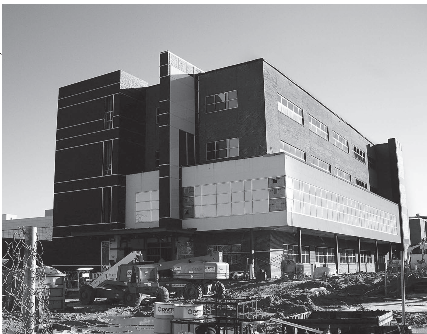
Independence-based contractor Frank A. Anzalone finished work on the $6.2-million expansion of the North Oaks Rehabilitation Hospital in the spring of 2007.
