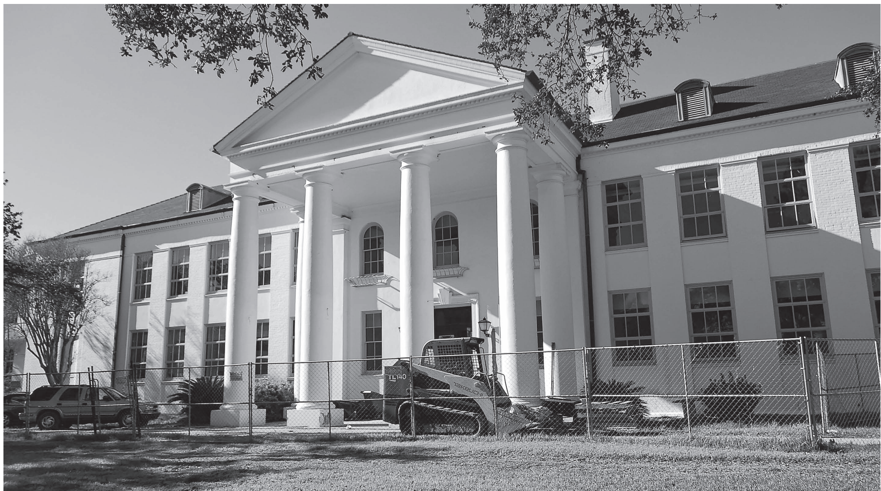
Repair work on Rosenwald Hall, one of the oldest buildings on Dillard University's campus, is expected to be completed by June when it will house the university's administrative offices.
