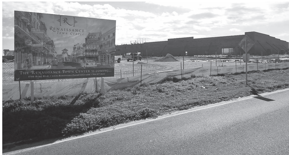
A Lowe's Home Improvement store under construction is the first component of an 80-acre redevelopment of the Lake Forest Plaza in eastern New Orleans.
