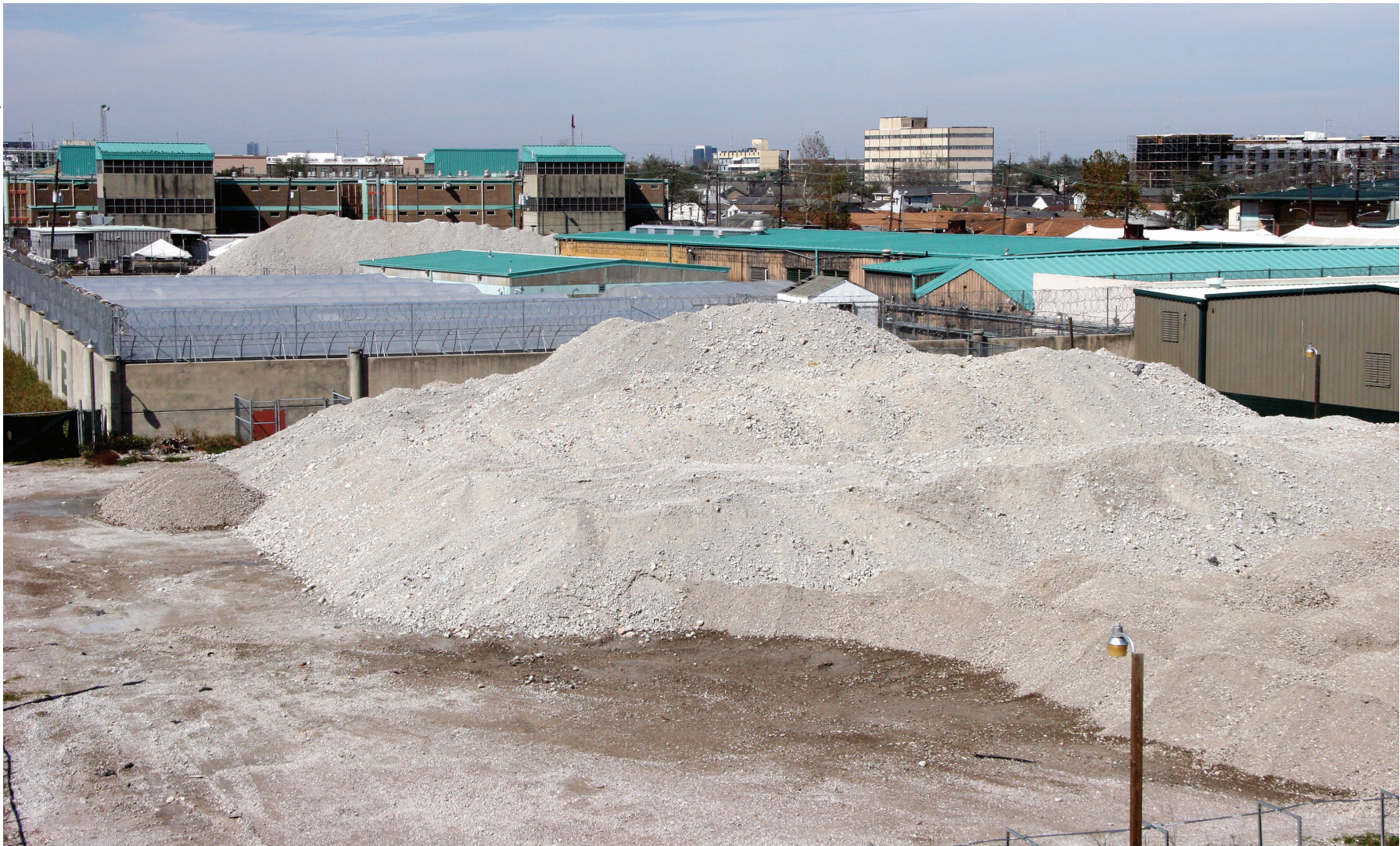
Site preparation has started for a new Orleans Parish Prison complex, which is expected to be completed by 2011.
