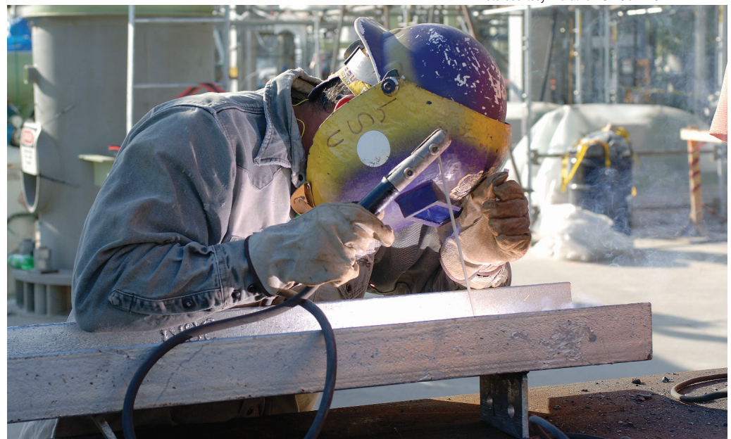
Work continues on the $3.35 billion Marathon Oil refinery expansion, which is expected to be completed by the fourth quarter of this year.
