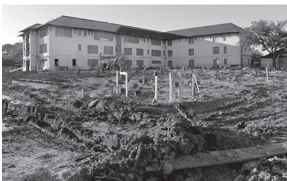
Andrew Wilson Elementary School is one of five Quick Start schools that will be the first new buildings in a $1.2 billion rebuild of Orleans Parish Public Schools.
