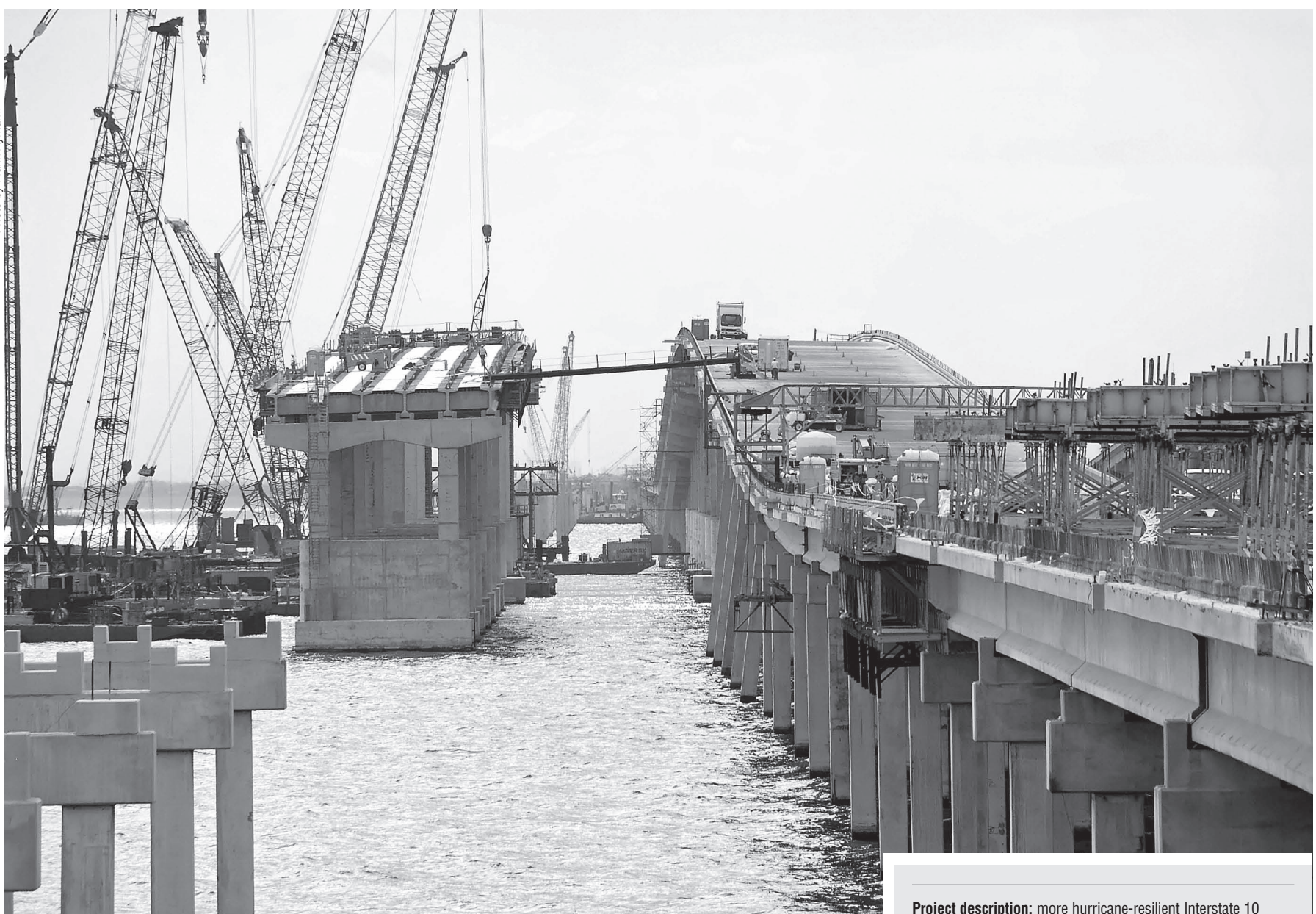
The Interstate 10 Twin Span, which was heavily damaged during Hurricane Katrina, is scheduled to open by August 2011.
