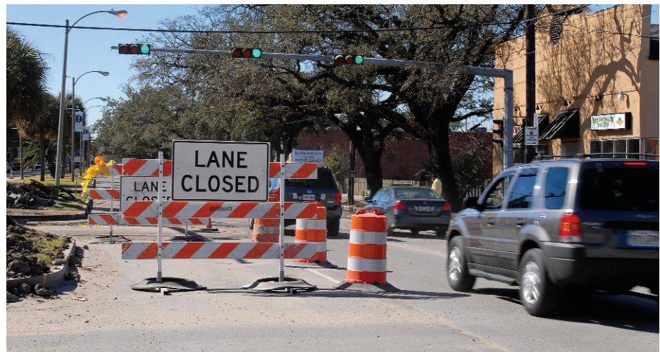
Traffic lanes are blocked during construction on Earhart Boulevard, a $12 million project that is expected to take a year to complete.
