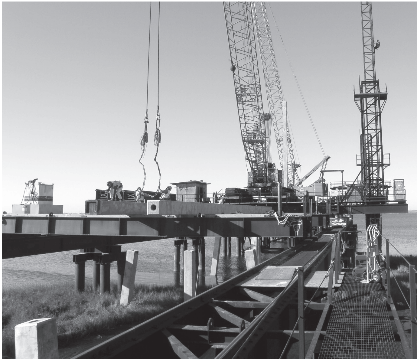
Work on a $150 million project to build a two-lane elevated highway south of the Leeville Bridge to Louisiana Highway 3090 is about 40 percent complete.
