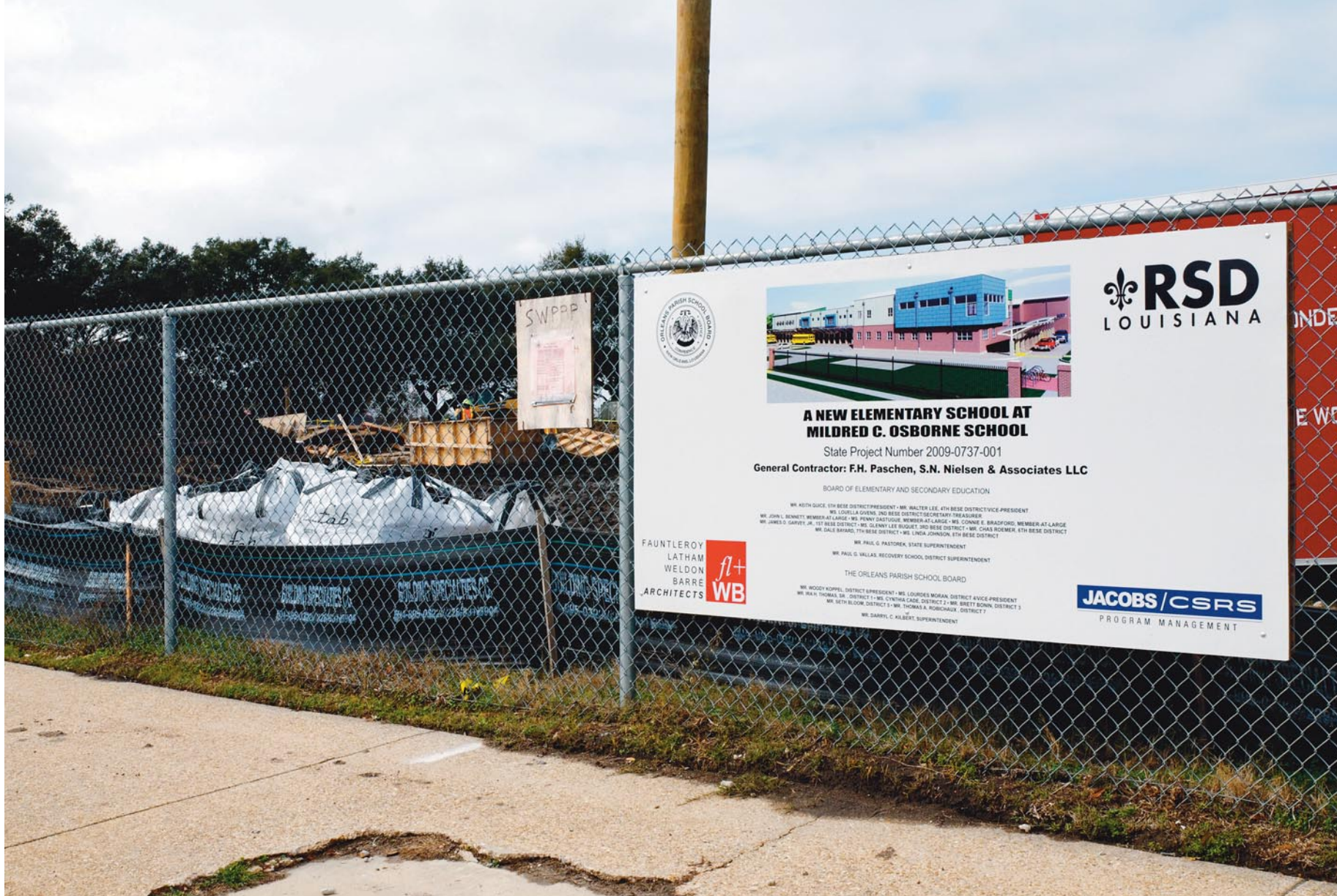
Site preparation is under way for the new Mildred C. Osborne Elementary School, one of seven public elementary schools under construction in Orleans Parish.
