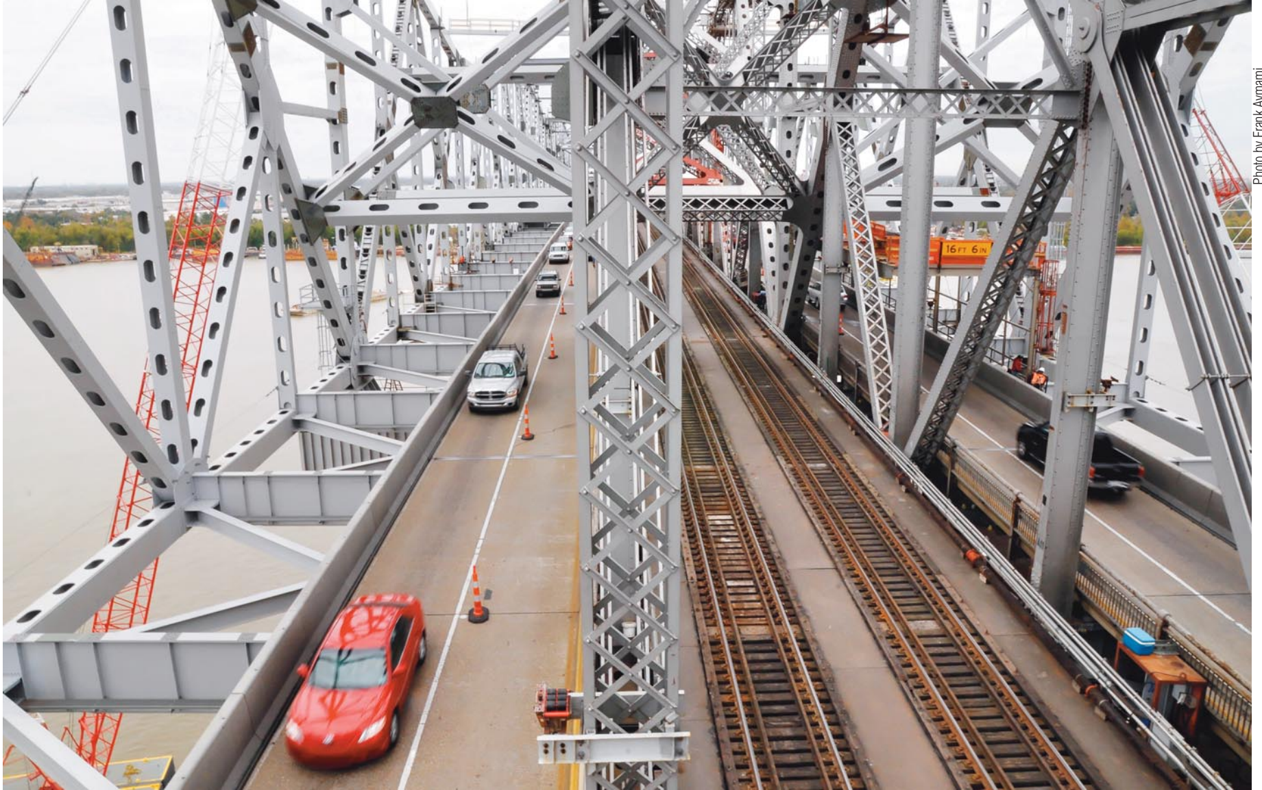
Officials expect to raise the final major piece of the Huey P. Long lane-widening expansion project into place in April.
