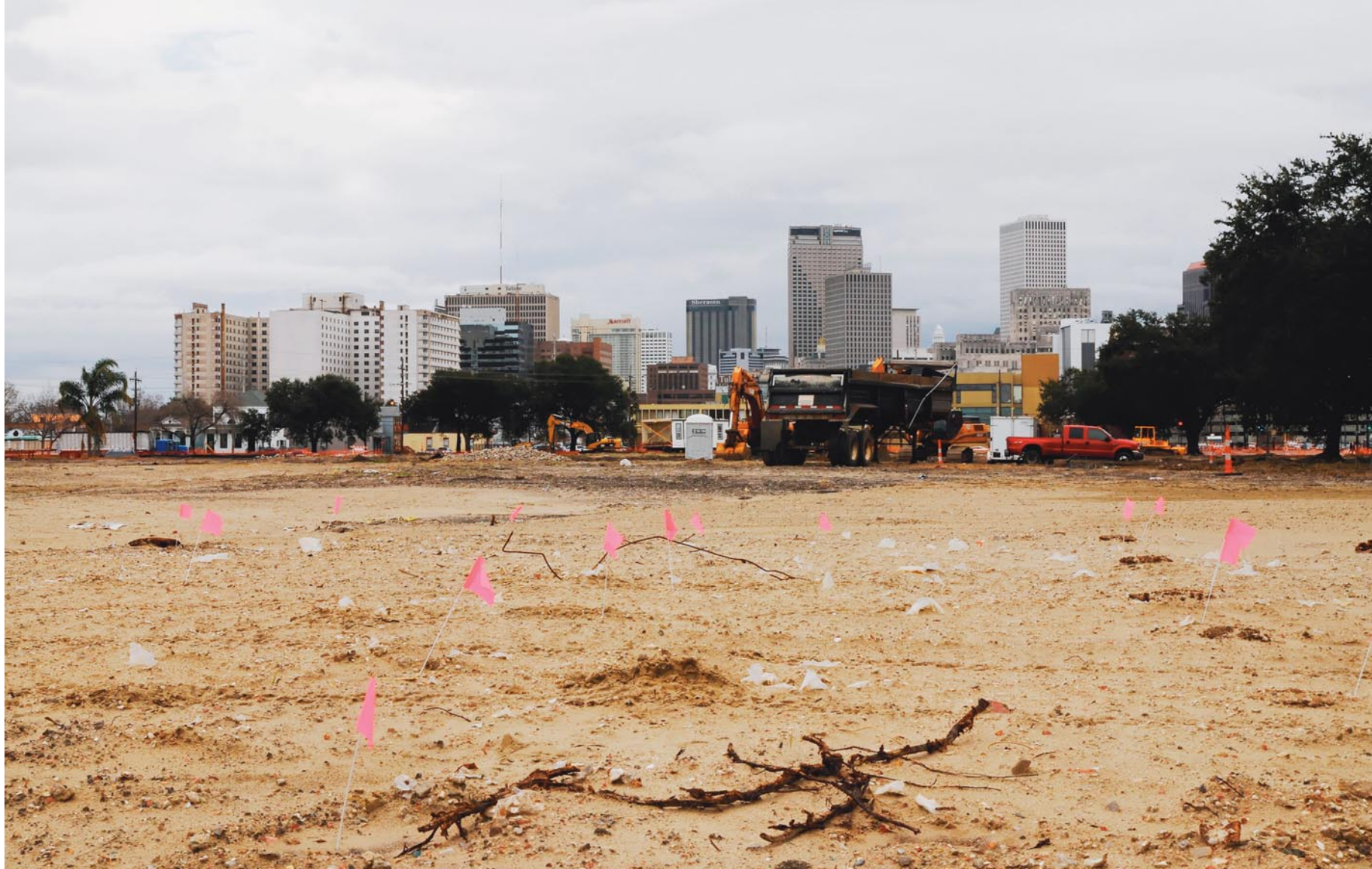
Crews continue to clear properties in the footprint of the new Veterans Affairs hospital, which is bounded by Canal, South Galvez and South Rocheblave streets and Tulane Avenue.
