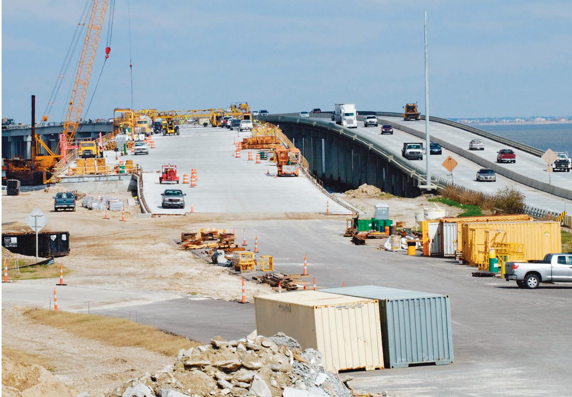
Work continues on the southbound onramps for the Twin Span, which is on schedule to open later this year.
