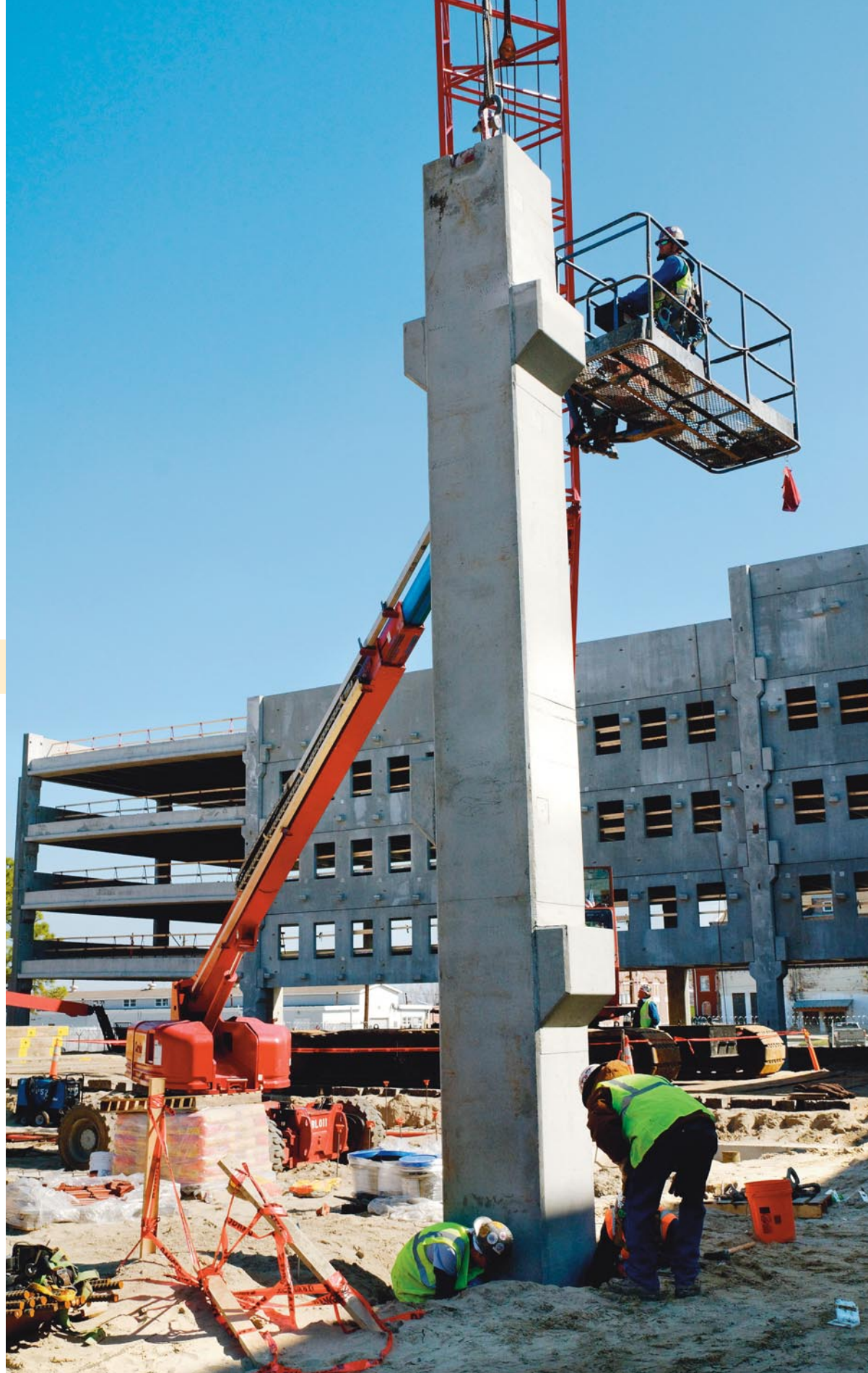
Workers install concrete pilings for the Federal City retail complex in Algiers.
