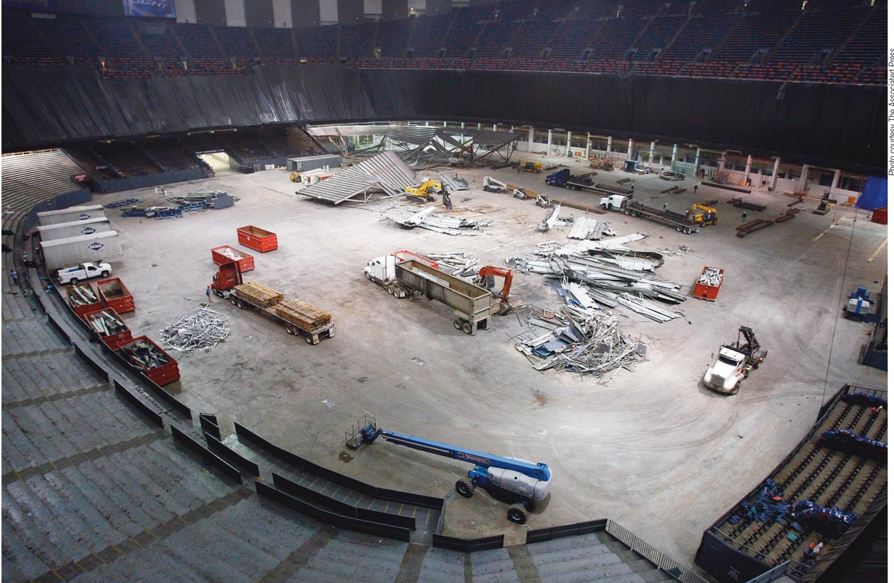
Workers demolish the Plaza Level of the Louisiana Superdome to make way for more premium seats, more concession stands and broader concourses.
