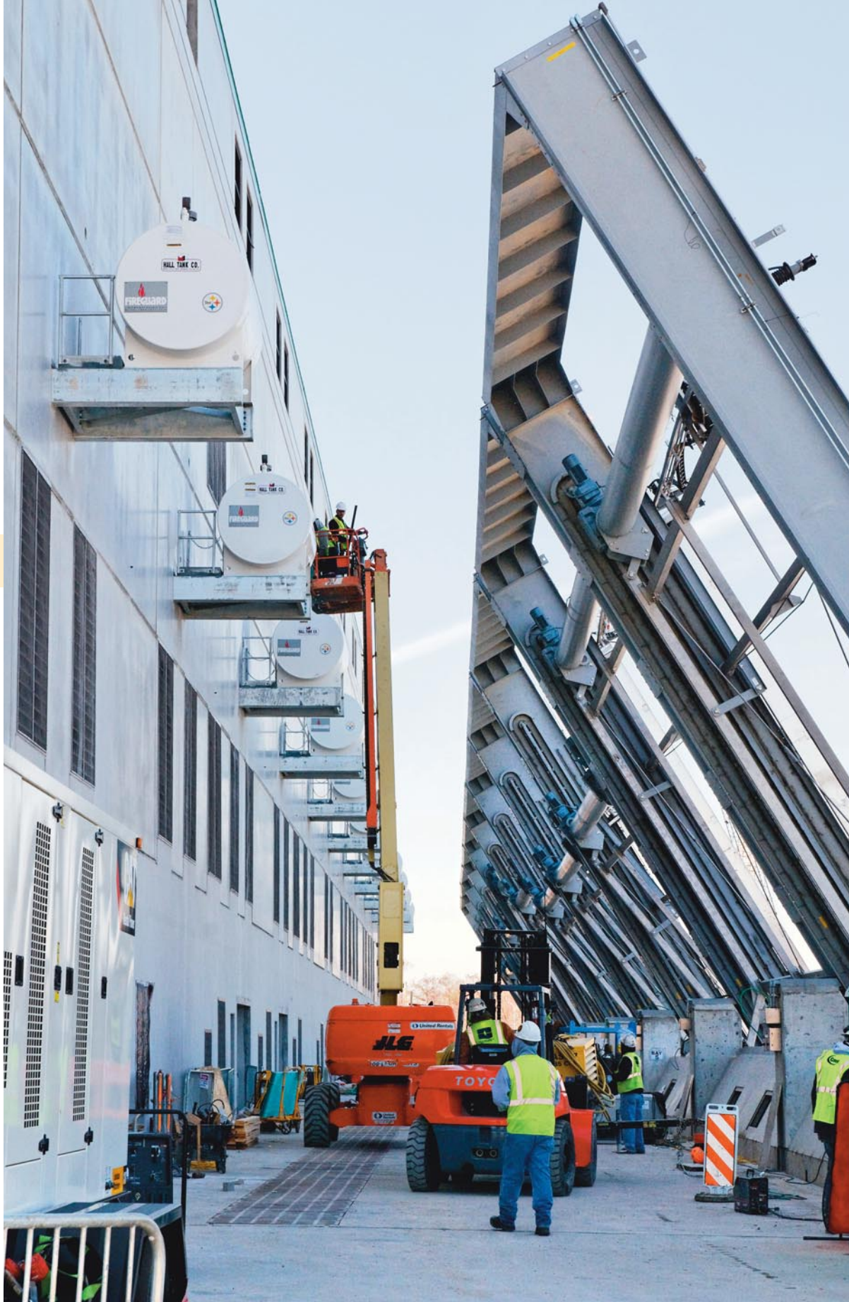
The U.S. Army Corps of Engineers is putting the finishing touches on the West Closure Complex in Belle Chasse. The pump station is the largest in the world and can empty enough water to fill an Olympic swimming pool in several seconds.
