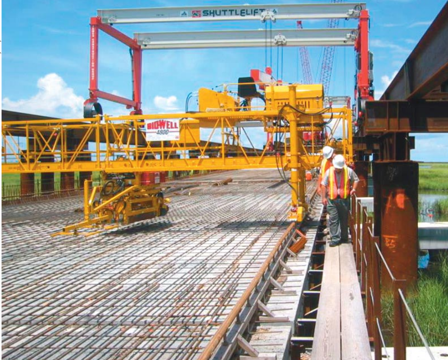
Work is expected to wrap up in September on a $150 million project to build a two-lane elevated segment of Louisiana Highway 1 from the Leeville Bridge north to Louisiana Highway 3090.
