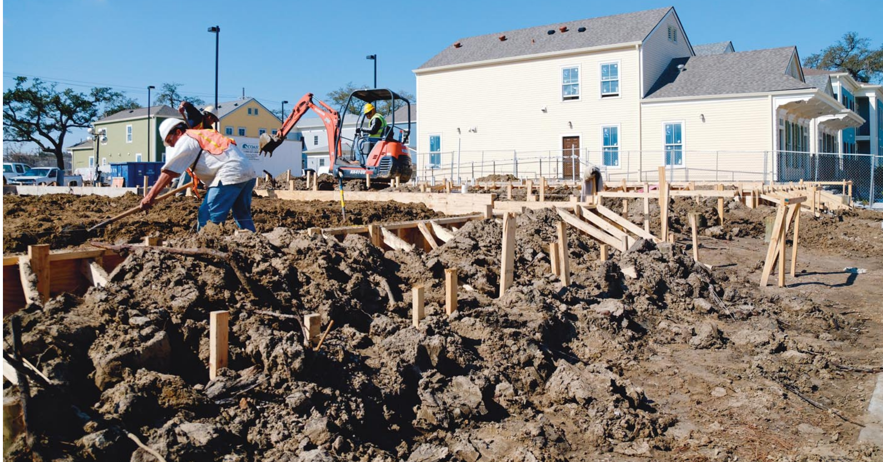
Workers prepare the foundation for the remaining 34 housing units at the Lafitte development, which is on track for completion this spring.
